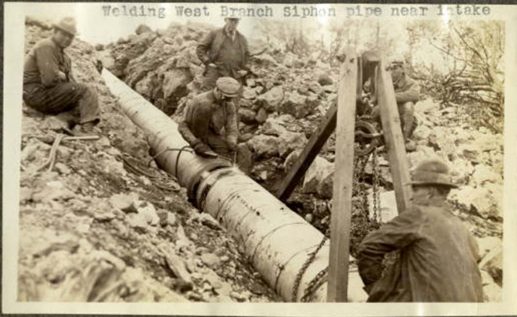
1924 Concow Dam Scrapbook Image 28b Caption: Welding West Branch Siphon pipe near intake
