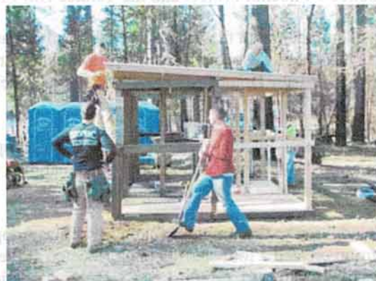
CONCOW RISING Chico State Construction Management students erect sheds for fire victims.
