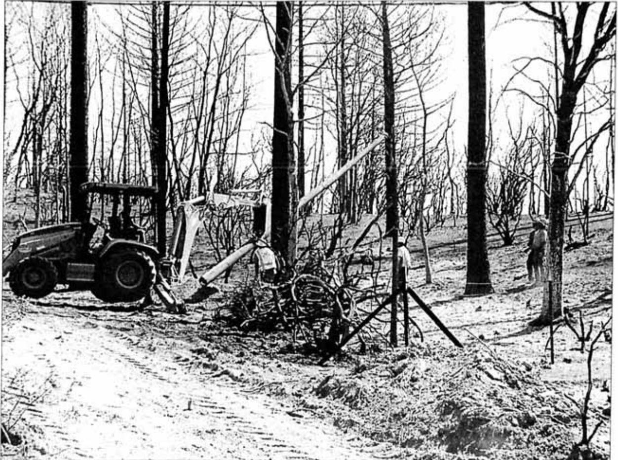
Utility workers were on the scene in some areas heavily hit by Friday's destruction. New poles were brought in to replace those damaged or destroyed as the fire tore through the Yankee Hill area.
