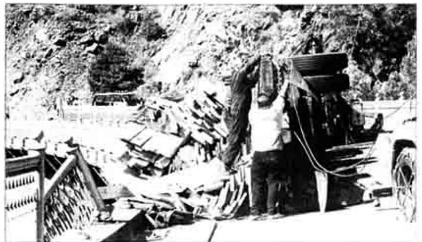
Two men wrapped steel cables around the trailer of a Sierra Pacific Industry rig and then used a larger wrecker to right it, in an attempt to open the Pulga Bridge. The road remained closed to through traffic from the time of the incident at 6:20 a.m. until it was finally cleared several hours later.
