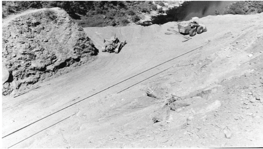
Feather River Canyon August 17, 1957 Milepost 229.1 Scene of slide three months earlier
